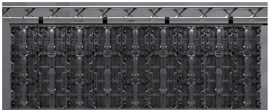
Video wall rear view / Truss hung
